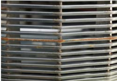
Stainless steel exterior light mast before treatment with Steel Brite cleaning systems
